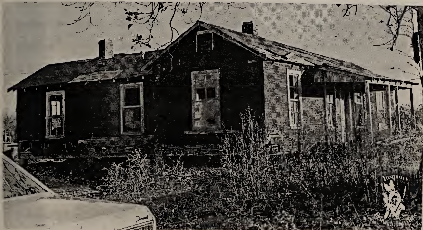
Plate 8. The only extant house in the Big Creek project area is this deserted example of the Balloon Frame method of construction. No. 1308-2
